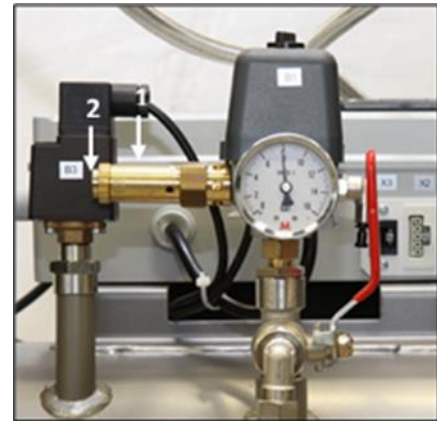
Fig. 17: Check of safety valve
